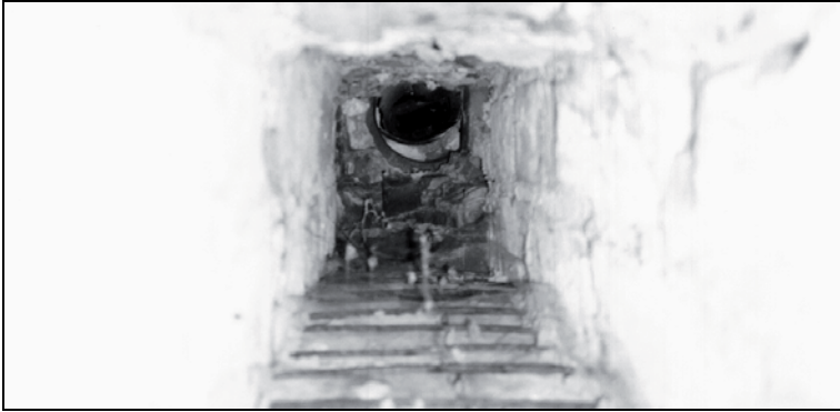
Photo 7: Delousing chamber at Stutthof, viewed from the south. The oven was used to heat the air inside the delousing chamber. Interior view of the combustion chamber. Beneath: the plane grid; above: the circular opening of the connection to the cast iron pipe located inside the delousing chamber. ©
