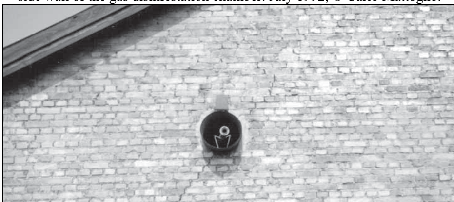
2. Birkenau, BW 5b. One of the two round openings for placement of ventilators in the outside wall of the gas disinfestation chamber. Above the sheet metal tube one can see, attached to it by means of a hinge, a metal plate to which the lid of the tube was welded. July 1992, © Carlo Mattogno.
