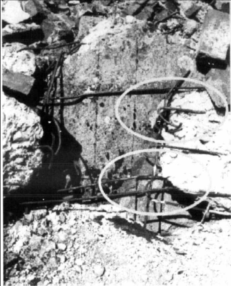
Figure 16. Remains of fourth (seen from south) Zyklon hole. Rebar skirts two sides, ends at other two sides bent inward and looped back. Note rotated roof slab showing formwork on inner side.
