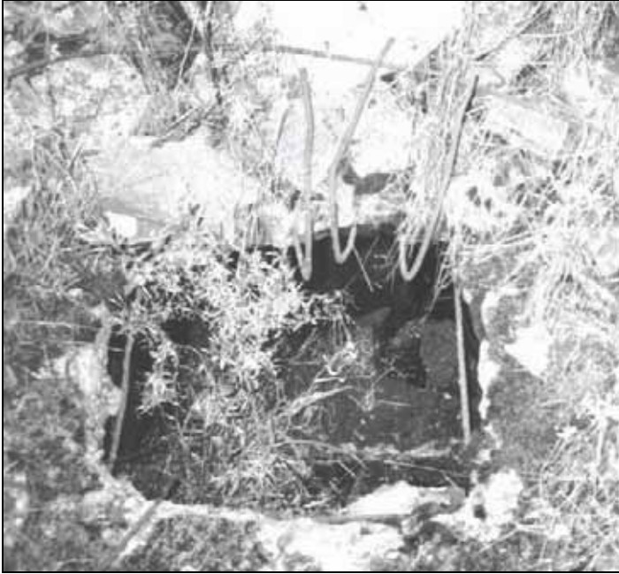
III. 25: Concrete roof of morgue 1 of crematorium II in Birkenau. Provan's opening 7 in October 1991. © Carlo Mattogno
