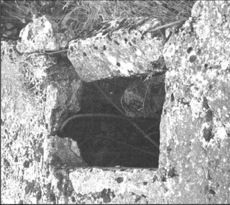
III. 13: Ceiling of the oven room of crematorium III. Second ventilation opening (seen from the west). June 1990. © Carlo Mattogno
