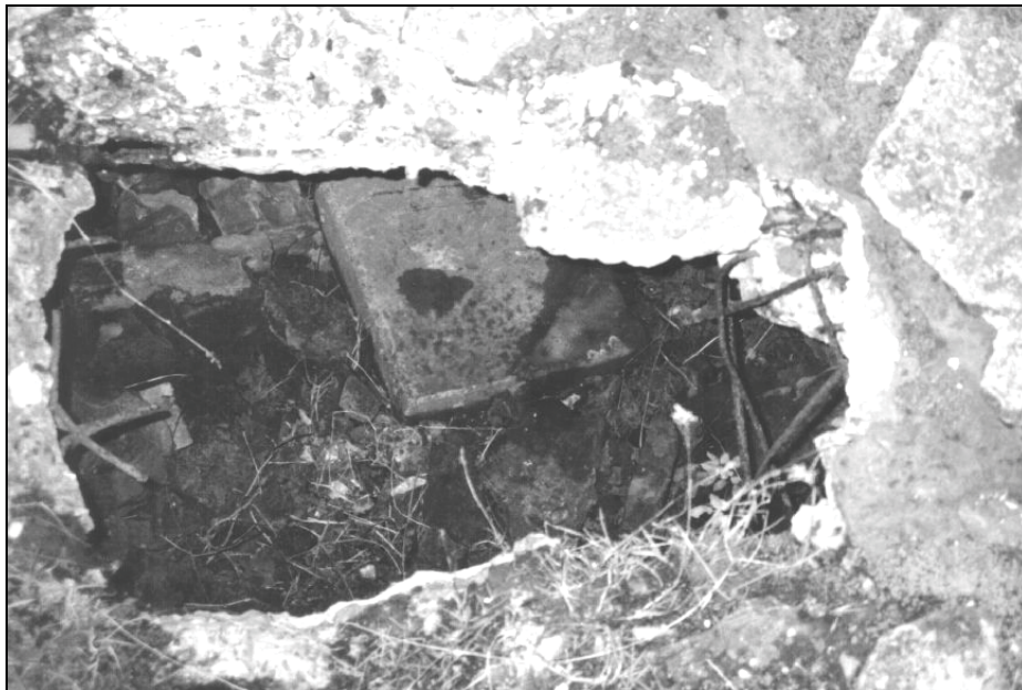
III. 29: Concrete roof of morgue 1 of crematorium II in Birkenau. Provan's opening 2 in October 1991. Inside the morgue on the floor a square concrete lid can be seen stemming from the sewer manhole of this crematorium. © Carlo Mattogno
