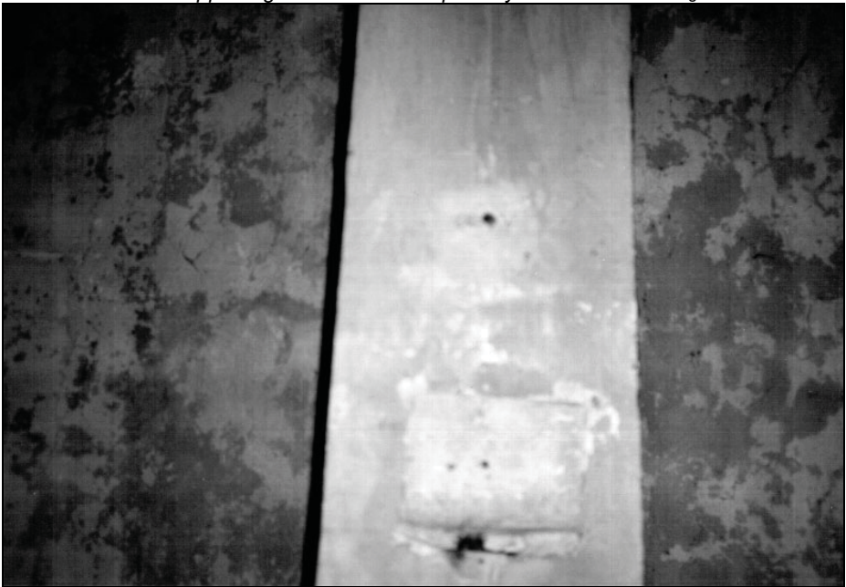
III. 12: Morgue of crematorium I at Auschwitz. One of the blocks set into the center of the supporting beam of the ceiling. October 1991. © Carlo Mattogno.
