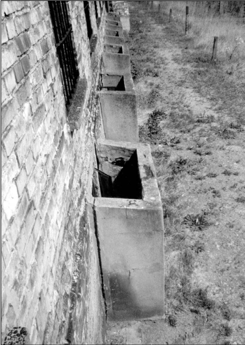
Photo 27: Block 11, wall facing SSW, closeup of concrete covers surrounding the windows of the Bunker cells. © Carlo Mattogno, Oct. 1991
