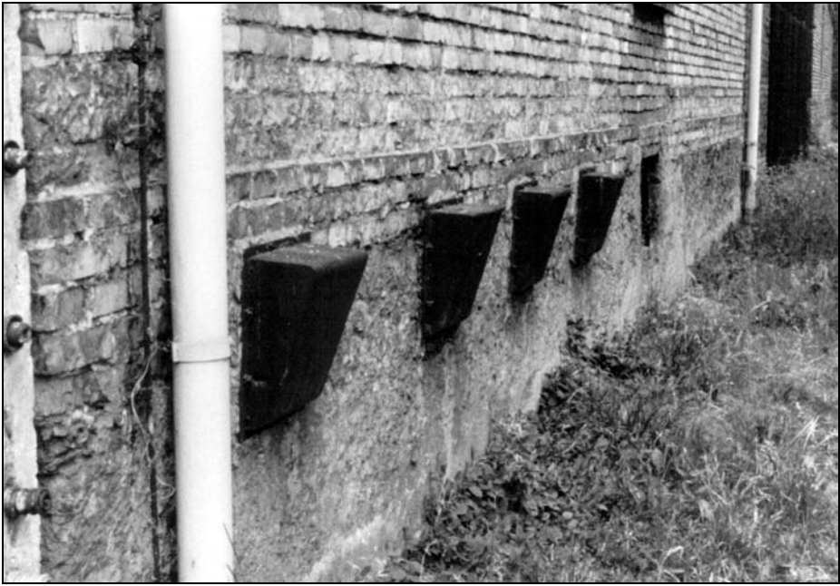
Photo 30: Block 11, outside, wall facing SE, sheet-metal boxes covering the air-supply holes of the 4 stand-up cells of the Bunker. © Carlo Mattogno, Oct. 1991
