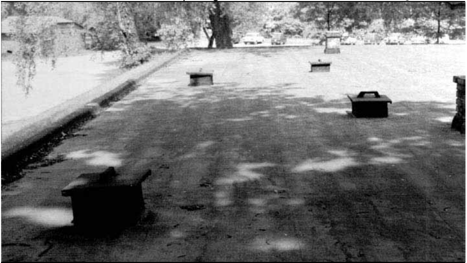
Document 23: Photo of the roof of the morgue. All four shafts constructed by the Poles after the war. © Carlo Mattogno
